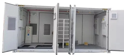
1075KW HH ESS
